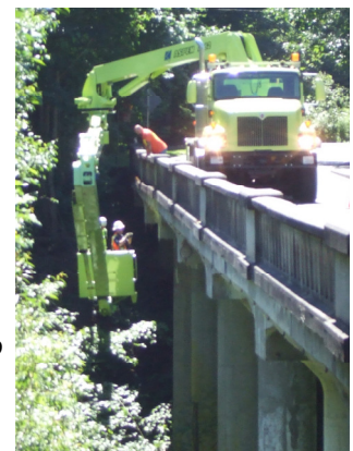
A bucket operator assists a Snohomish County bridge engineer during the bridge inspection.
